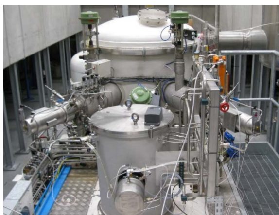
Fig. 1. Cold Box ALPI. In front is the supercritical Turbine
